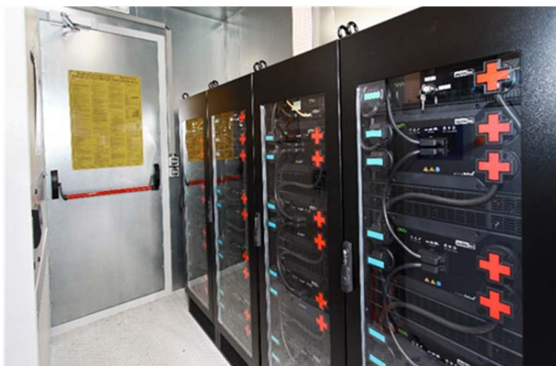
The batteries store solar power and feed it into the mains of HIU, if required. (Photo: Frederik Elschenbroich, ads-tec)
